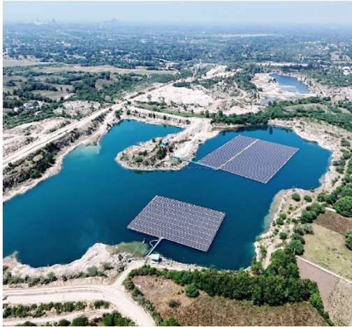
Developed a floating solar plant at Daroli Mines, the first in India's cement industry
