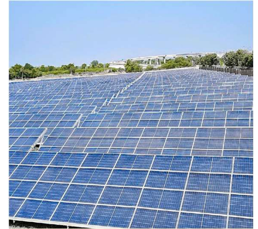
Commissioned Rooftop solar project in Uttarakhand
